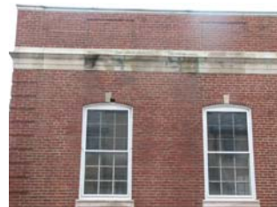
Missing Masonry Above Window
